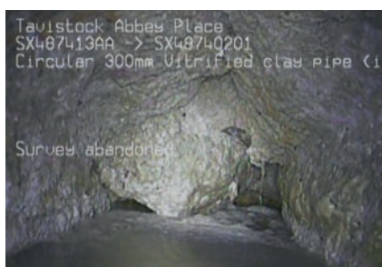
CCTV survey showing fat build up in a sewer
