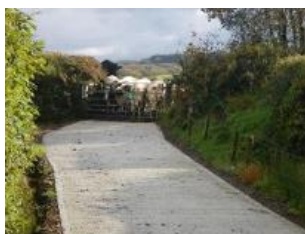
Track and cross drain works completed on River Deer to prevent sediment run-off – photos before (top) and after (bottom)
