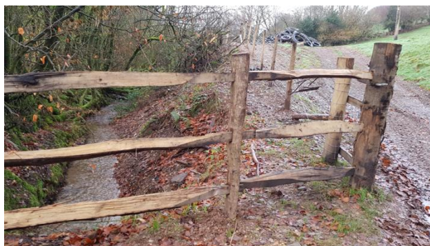
New fencing to protect the banks from livestock erosion and faecal contamination
