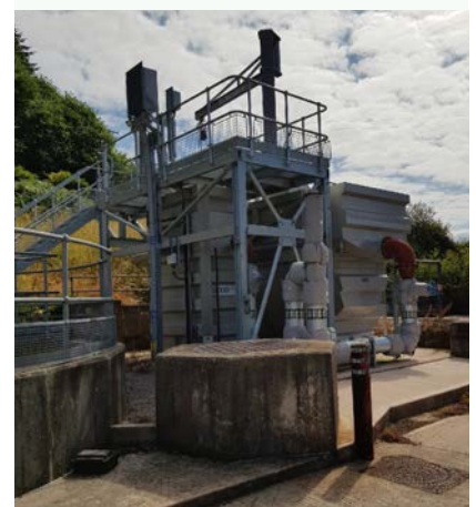
Top Reactive media reed bed (Wilmington), Above Mecana cloth filter with flocculation tank (Kenn & Kennford WWTW)
