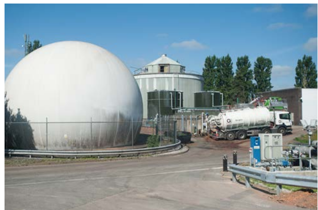
Combined Heat and Power facility, Countess Wear
