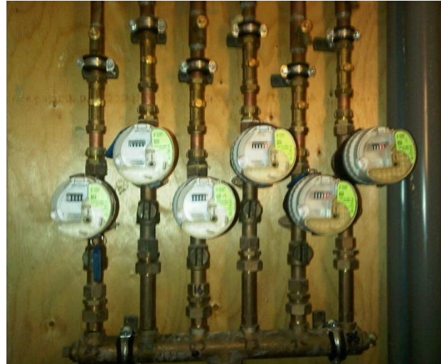
Manifold and Meters
